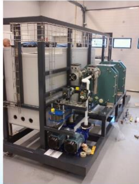
Test unit in Qatar. Treatment of produced water (contaminated water from oil and gas exploration ) at the Global Sustainability Center (GWSC) at Qatar Science & Technology Park (QSTP).
