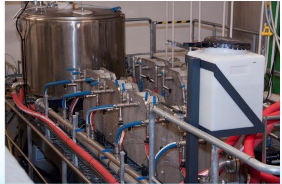
Test and demonstration installation at Sjöstadverket in Stockholm
